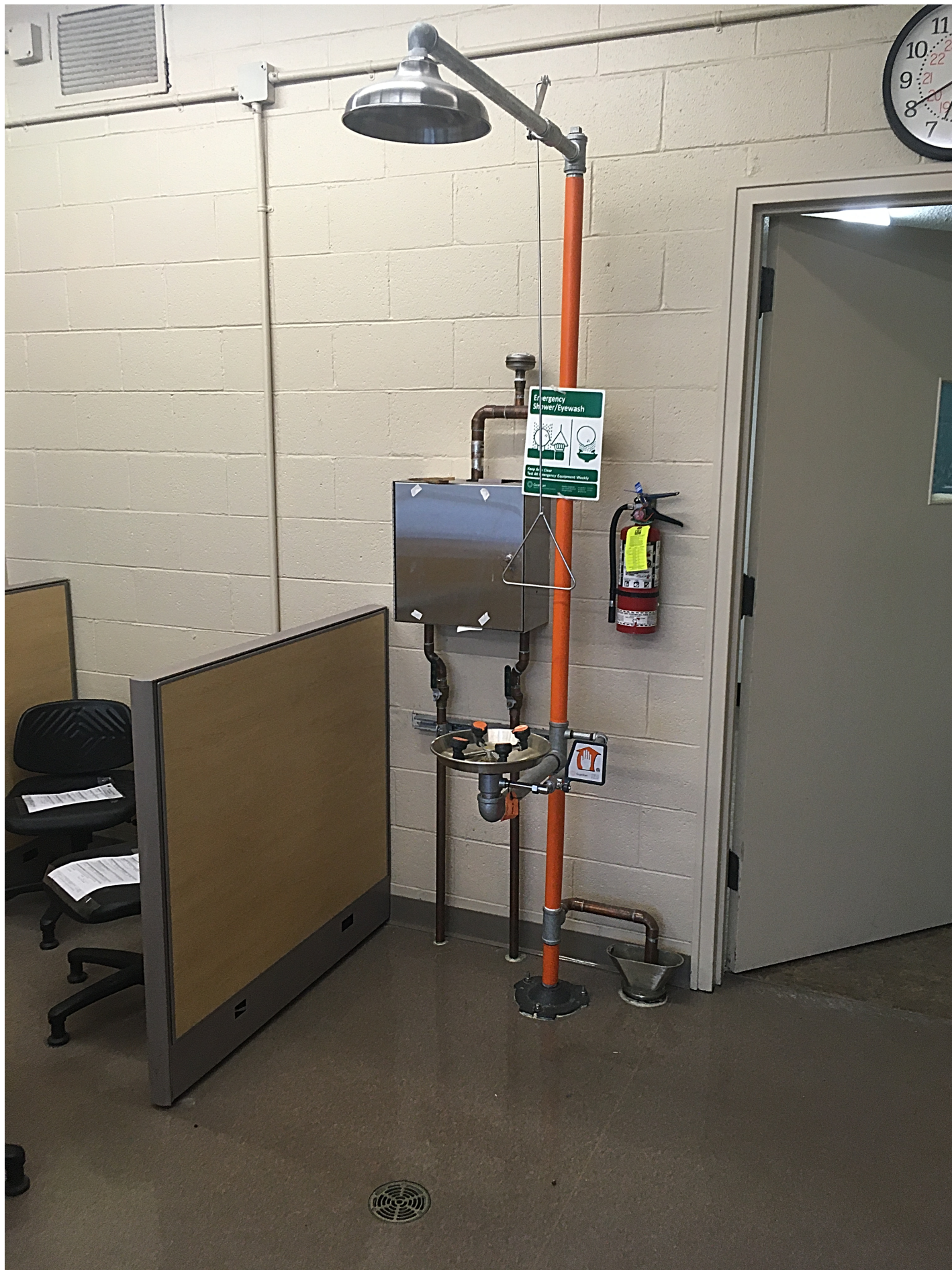
SCIENCE BUILDING, SN-3123 COMBO EYE/FACE WASH AND SHOWER STATION
