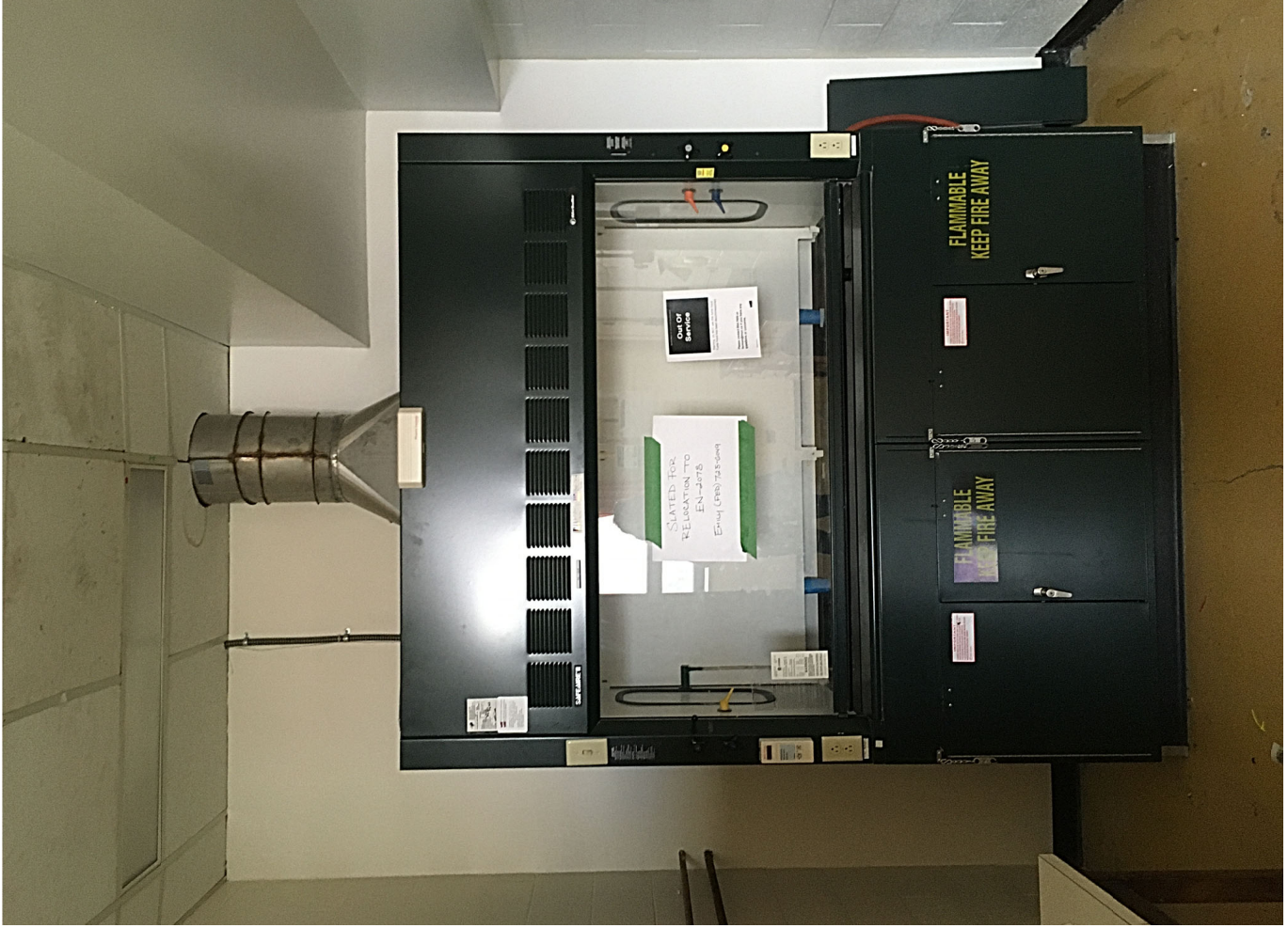
CHEMISTRY-PHYSICS BUILDING, C-5006A FUMEHOOD
